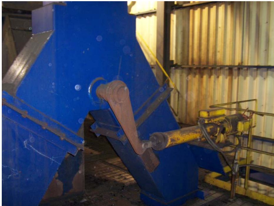
Figure 3 The variable position diverter is used to determine the percentage of raw coal which will bypass the prep plant.
