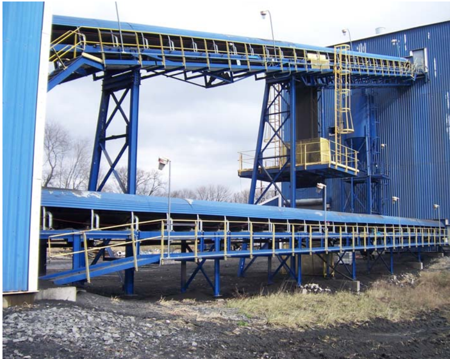
Figure 4 The top belt is prep plant feed. The bottom belt is prep plant bypass.
